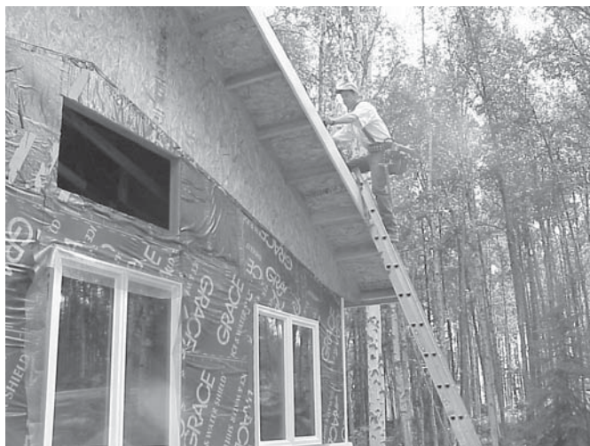
Figure 7. Roofed PERSIST home which used Grace Ice and Water Shield® as the air-vapor retarder on the exterior skin. Hébert prefers bituthene now, as its adhesion and application simplicity are both superior to Grace Ice and Water Shield®. This photo shows the structure relatively complete, with only the 4 inches of exterior expanded polystyrene insulation and stucco finish to be added.
