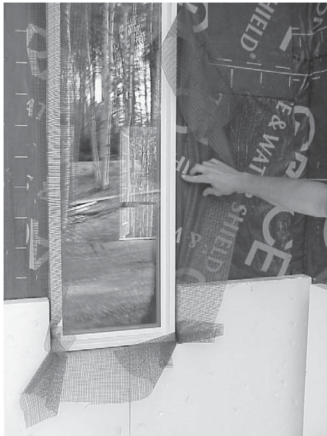
Figure 6. A window detail in a PERSIST home. PVC windows are flashed and sealed to the structural exterior sheathing. The mesh is a base for applying a final exterior finish of stucco.
