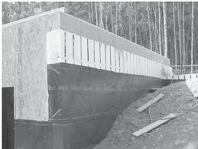
Figure 5. Foundation damp-proofing over ICF (insulated concrete form) system used by Jack Hébert in construction of his latest PERSIST type of home construction. In this case, the below-grade water/damp-proofing is bituthene, which is very self-adhesive and a very good practical choice.
